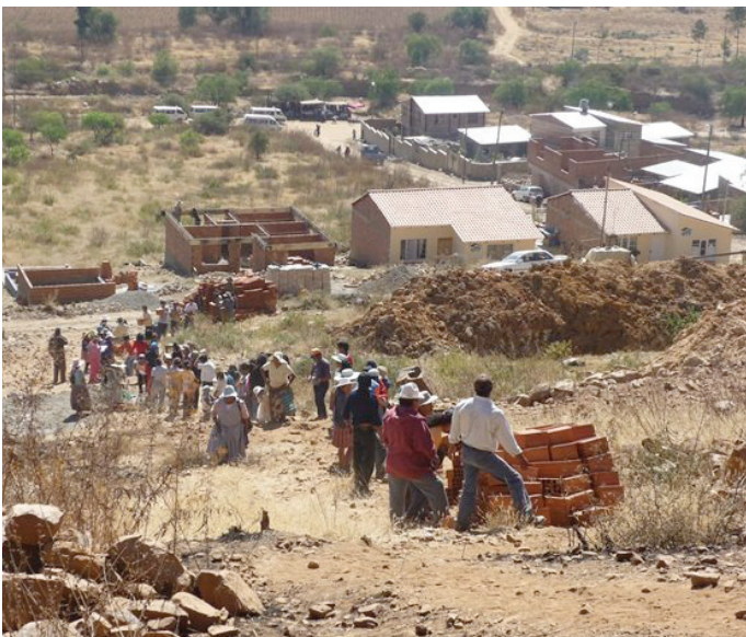
Residents form a line to transport bricks up a hill for the construction of a house in the Maria Auxiliadora community in Cochabamba, Bolivia.
